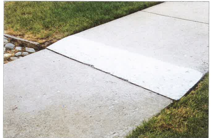
After Precision Concrete Cutting has completely and smoothly removed the trip hazard.
