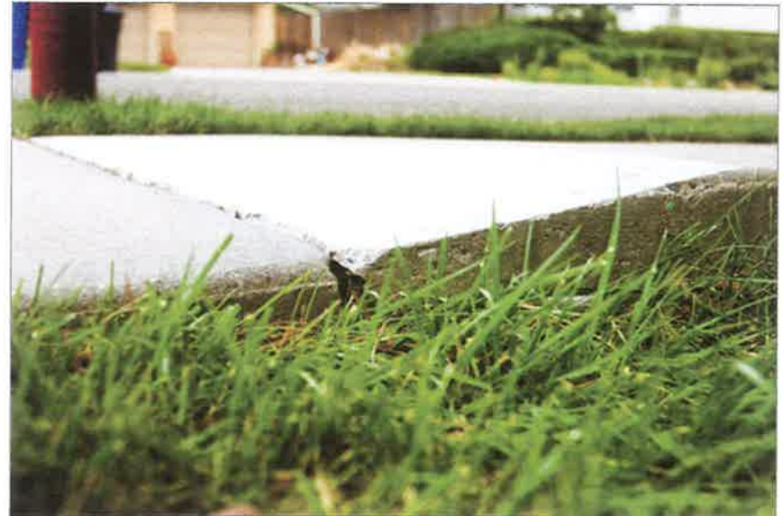
After Precision Concrete Cutting has completely and smoothly removed the trip hazard.
