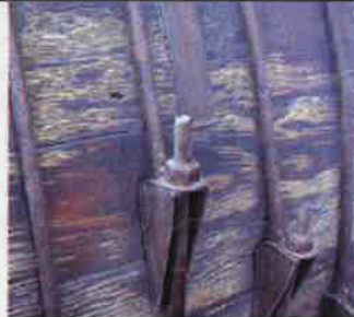
Old wooden pipes are a unique feature of the King County sewer system.
