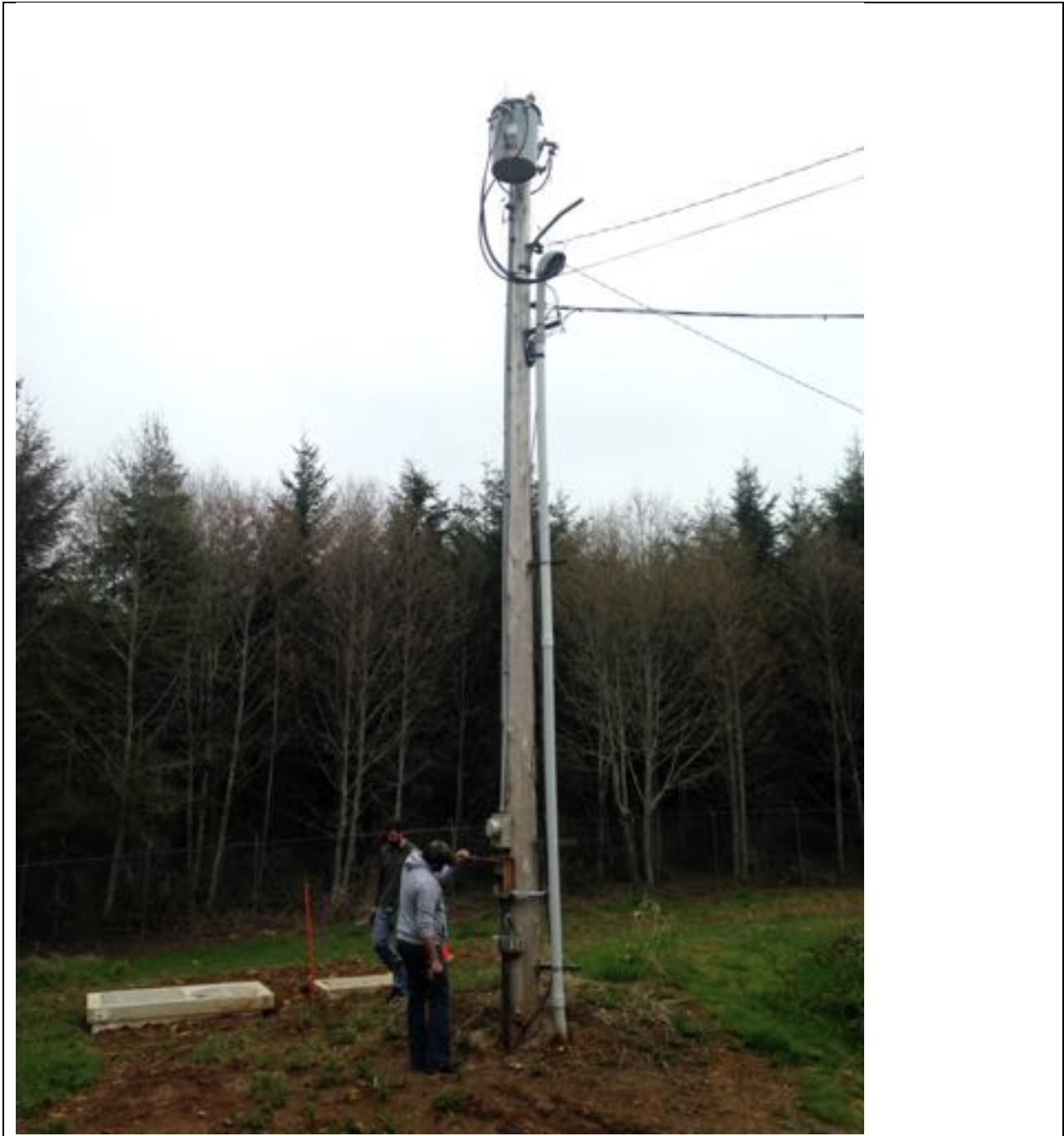
Image 2. Electrical Meter at Reservoir Site
