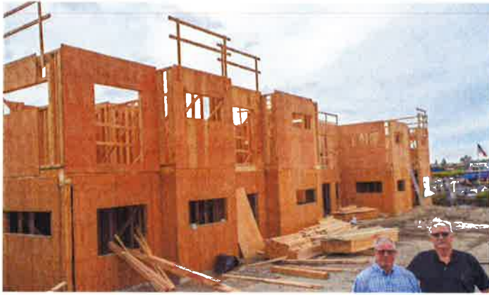
iStudios North is a multi-unit apartment development being built near the Tacoma Mall by Steve Novotny (left) and Roy Kissler, October 3, 2016. Peter Haley - phaley@thenewtribune.com
